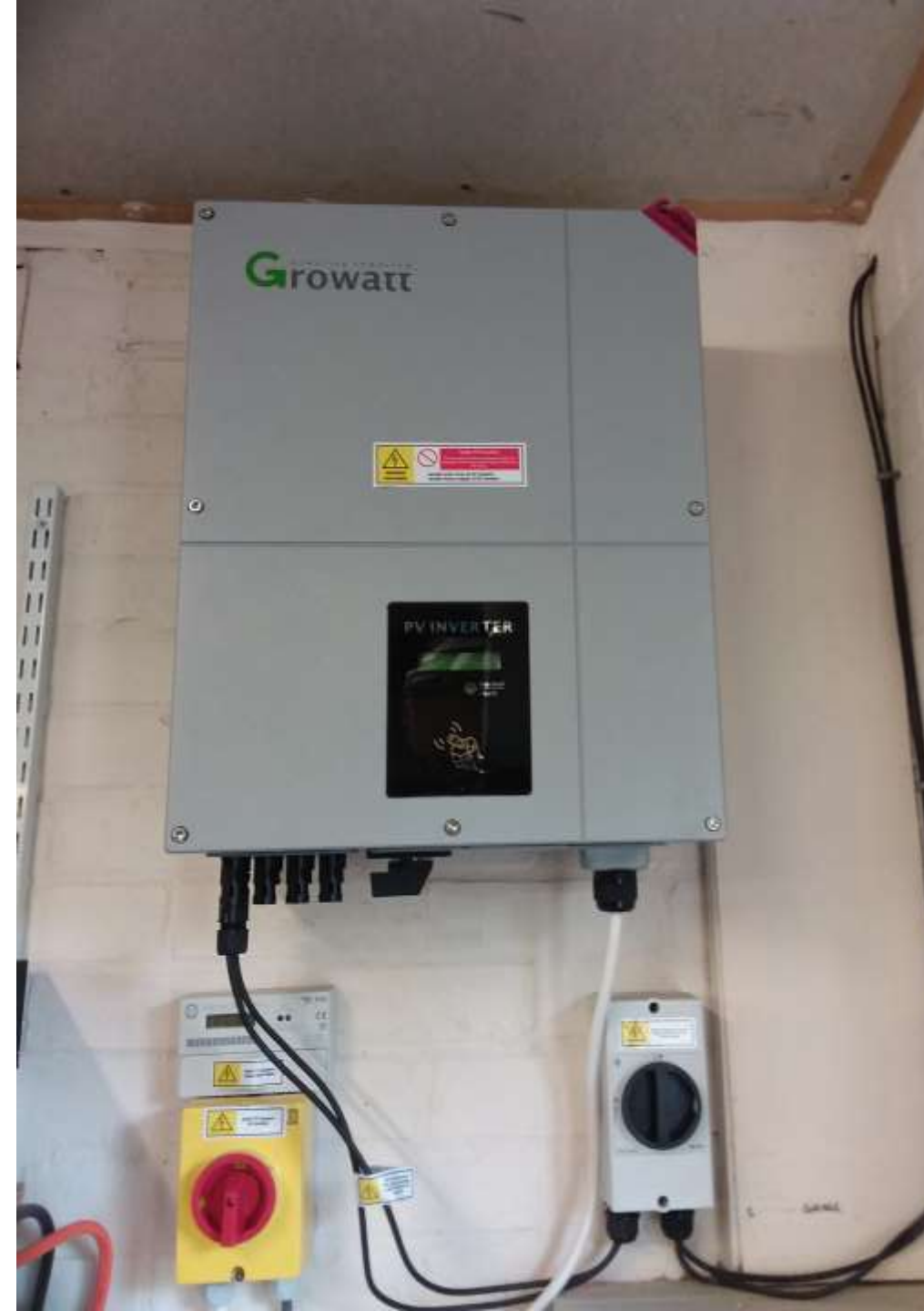
Inverters for the Solar PV
